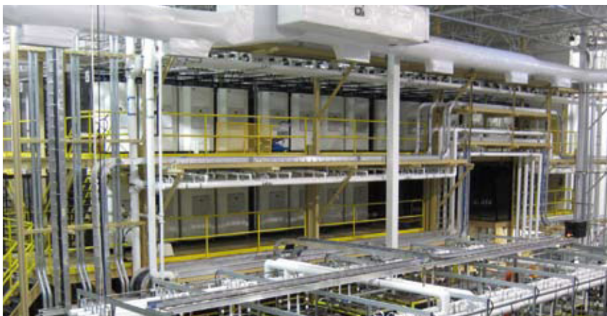
Above: Automation of all processes - formation, degassing, ageing, grading, sorting
